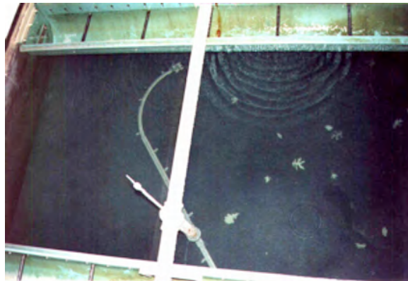
GAC-Capped Filter, Bloomington, Illinois
