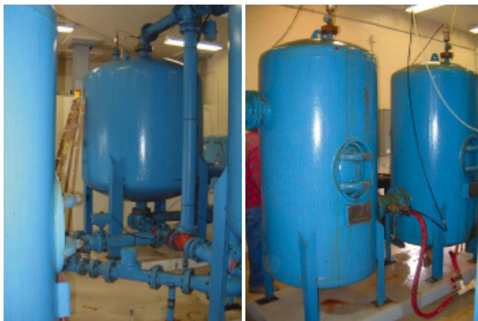
Filtronic's Filter Units and Reaction Vessels
