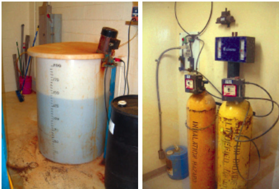
Ferric Chloride and Sulfur Dioxide Feed Systems
