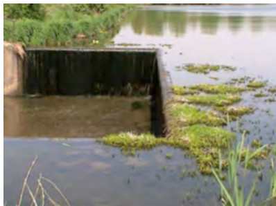
Algal Growth and Vegetation at Lake Spillway
