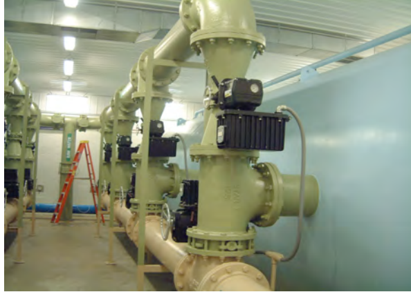
Horizontal pressure filters are divided into four compartments containing dual, crushed anthracite coal and coarse sand, media
